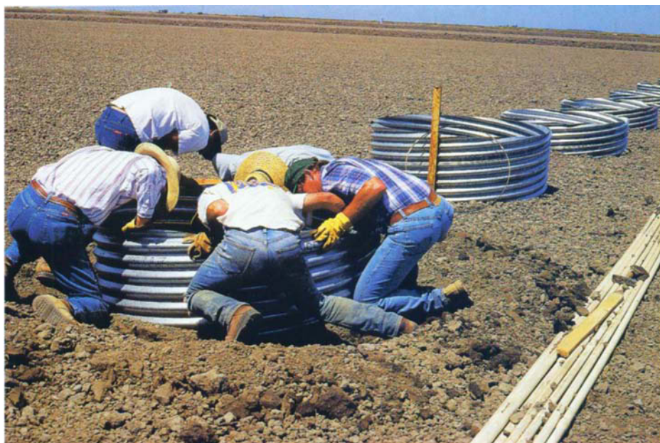
UC scientists install the rings into a grower's field to the depth of the plow pan, about 4 to 6 inches. Rice was then sown and cultivated in the fields as usual by growers, while researchers flooded the rings with water at various salinity levels.
